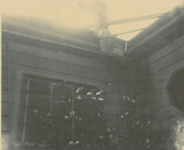
Mr. L. G. Meisner, installing new roof at their home, 4048 N. Haight
