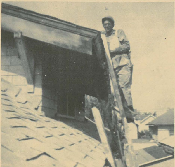
Installing roof and gutters on home of Mr. and Mrs. Willie Smith - 3513 North Commercial
